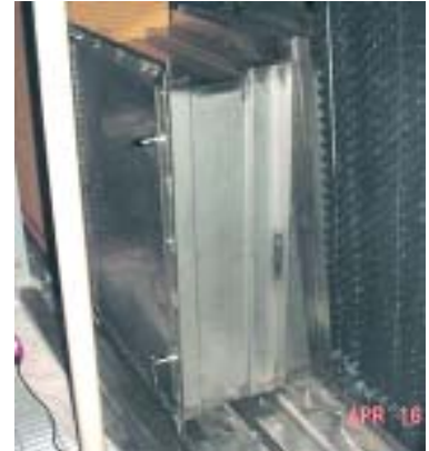
Here you can see the depth of the 'hobbit' door access hatch.
