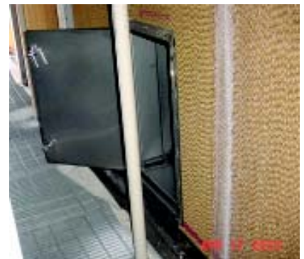
The 30"-high 'hobbit' door opens easily for access to the transition area behind the evaporative cooler media.
