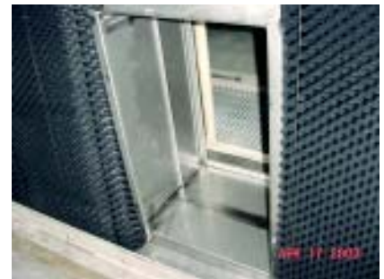
From the backside. The drift eliminator panels snug up to the sides of the door.
