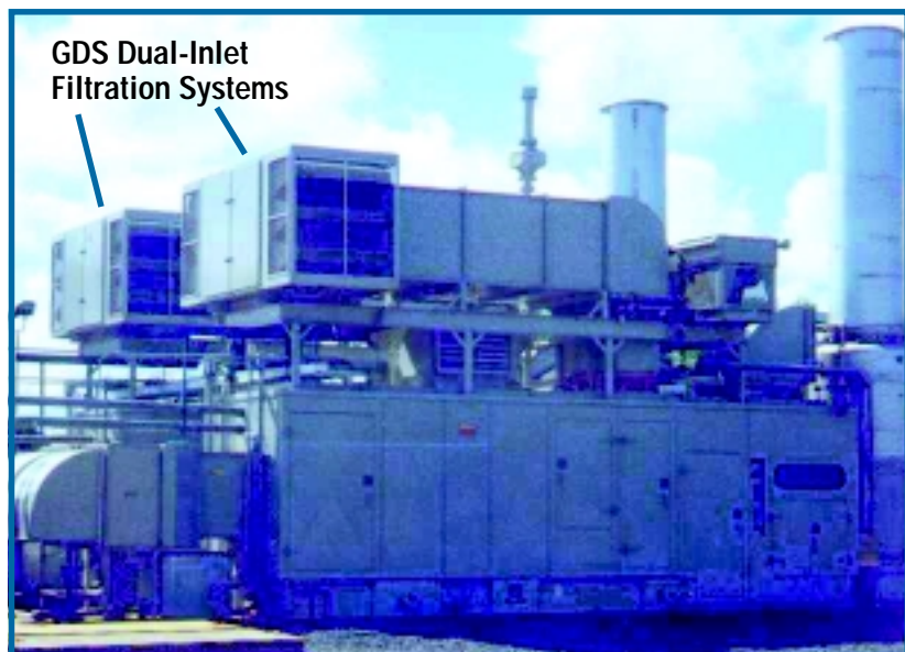
These Donaldson Dual-Inlet GDS Filter Systems protect turbines from the ravages of sand and dust near Tucson, Arizona USA. Note the insect screens over the inlet hoods. Donaldson GDS systems keep combustion air clean for hundreds of turbines all over the world.
